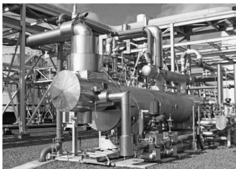
Fig. 8 Appearance of IFV for supplying cold energy to air conditioning apparatus in Kagoshima Terminal of NIPPON GAS Co., Ltd.
