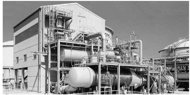
Fig. 4 Appearance of LNG cryogenic power generation plant in Osaka Gas Co., Ltd.
