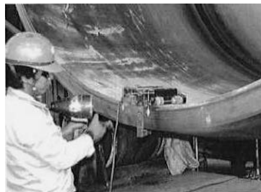
Photo 4.1 — Magnetic particle testing of the bevel surface of a welding joint with a heavy section
