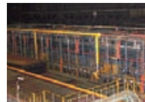
New heat treatment furnace
