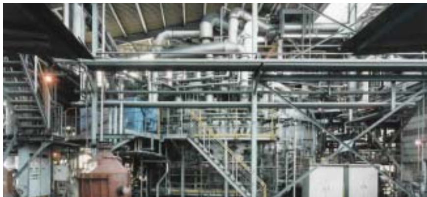
This FASTMET® Direct Reduction Plant contributes to zero emission activities at Kakogawa Works by reclaiming zinc-rich iron oxide dust from blast furnace and steelmaking operations.
