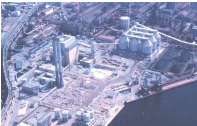
In 2004, we will have the capacity to generate 1.4 million kilowatts of electricity at Kobe Works. With trial runs underway at the No. 1 Power Plant, construction is proceeding on the No. 2 Power Plant.
