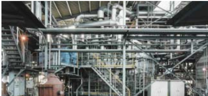
This FASTMET® Direct Reduction Plant contributes to zero emission activities at Kakogawa Works by reclaiming zinc-rich iron oxide dust from blast furnace and steelmaking operations.
