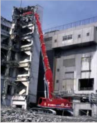
■ The SK 1600D can demolish buildings over 50 meters tall. The ultra long boom gives this machine one of the highest reaches in its class.
