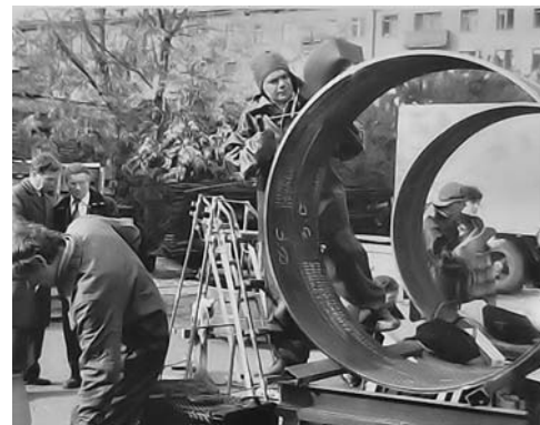
Figure 12: Welding test of covered electrodes on pipeline segments in the then Soviet Union in 1982.
