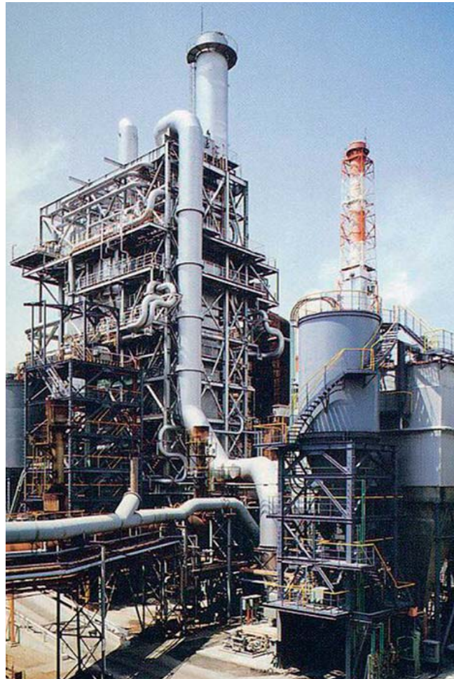
燃煤火力发电厂 Coal-fired Steam Boiler Plant
