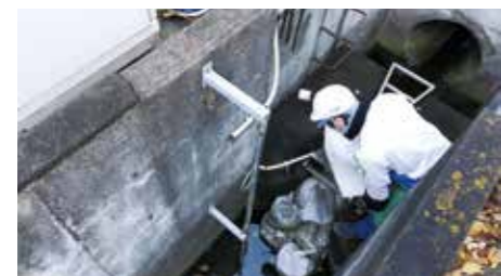
Drill on setting out sandbags and oil absorbent mats in preparation for leakages (Shinko North Co., Ltd.)
