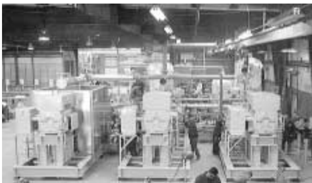
Photo 1 Screw compressor for gas turbine fuel gas
