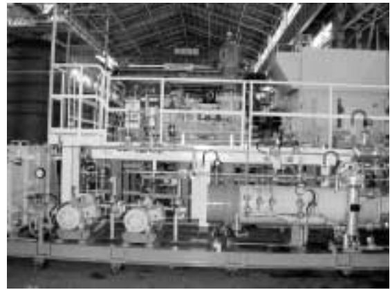
Photo 2 Screw compressor for desulfurization process
