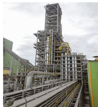
Fig. 5 Latest MIDREX NG plant: Tosyali in Oran, Algeria. (Reduction furnace in center with HDRI conveyor to EAF meltshop on left side.)
