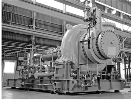
Fig. 6 Centrifugal compressor for PDH application
