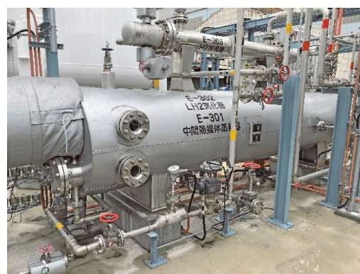
Fig. 2 Outside view of IFV for LH 2 vaporization demonstration
