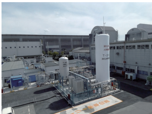
Fig. 4 Outside view of LH 2 vaporization demonstration facility
