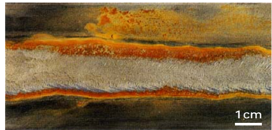
Figure 1: Rusty appearance of a weld bead after brushing with a carbon steel wire brush
