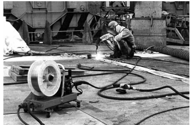
Figure 3: FCAW of stainless-clad steel butt joints in the inner bottom plates of a cargo tank
