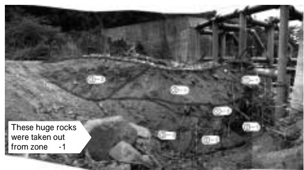
写真3 ダム上流部における堆砂縦断面図(中谷川砂防ダム) Photo 3 Vertical section of sediment at upper stream of the dam (The Nakatanigawa sabo dam)
