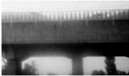
写真3 新幹線用山形防音壁 Photo 3 Mountain shaped barrier alongside super express railway
