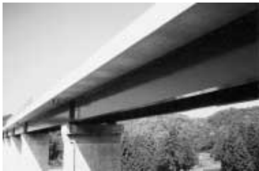
写真2 2主桁橋梁(儀明川橋) Photo 2 Two I-girder steel bridge (The Gimyogawa Bridge)
