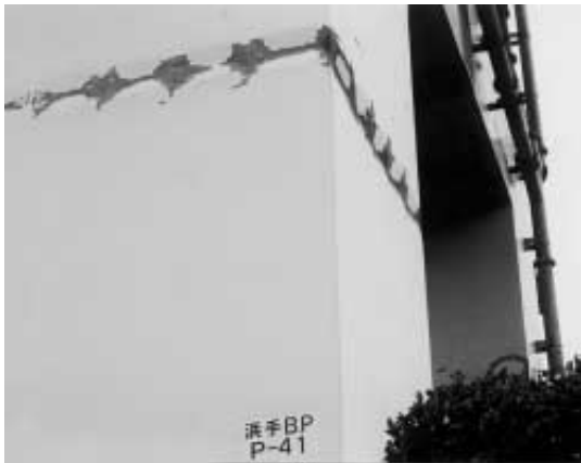
写真3 阪神・淡路大震災による鋼製橋脚の座屈 Photo 3 Buckling of steel pier by Great Hanshin-Awaji Earthquake Disaster
