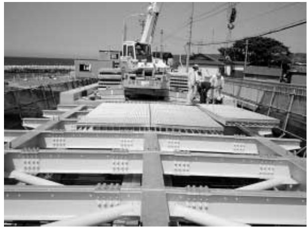
写真3 今別橋架設状況 Photo 3 Construction of open grid deck (The Imabetu Bridge)
