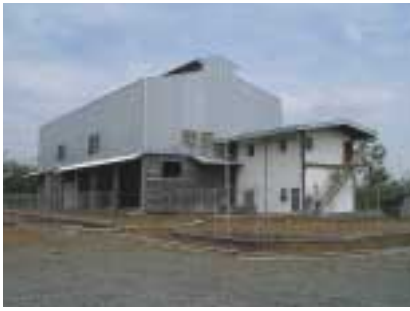
写真3 建設中の UBC 実証プラント (5t/d) Photo 3 Pilot plant of the UBC process under construction (5t/day, Cirebon)
