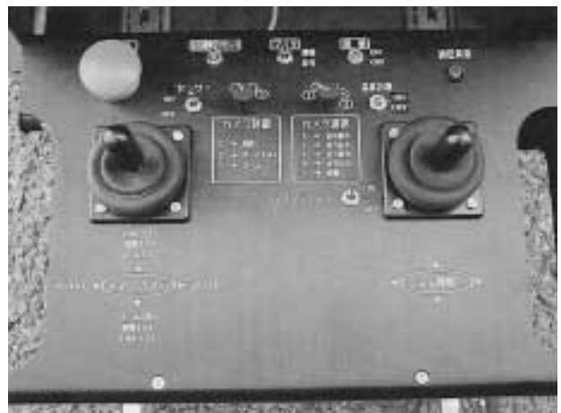
写真3 集中操作卓 Photo 3 Concentrated control panel
