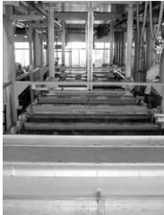
写真2 抗菌めっき処理ライン外観 Photo 2 Photograph of anti-microbial electroplating equipment
