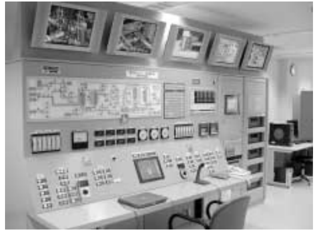
写真4 計測制御室 Photo 4 Control and data acquisition room
