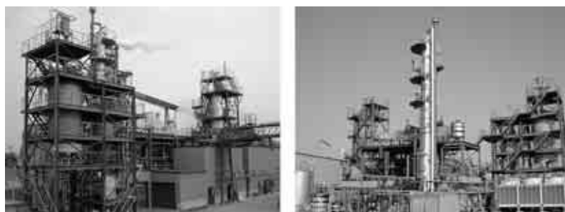
写真1 脱塩素処理設備全景 Photo 1 De-chlorination facilities in Kakogawa Works
