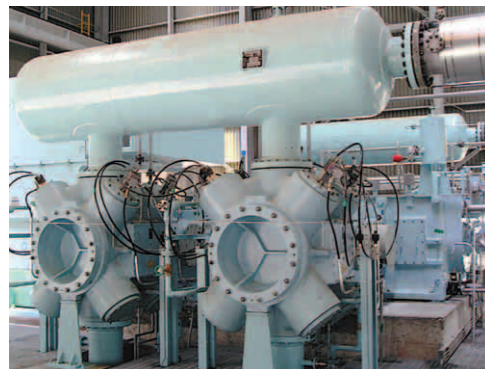
図2 KR60-4 無段階容量調整装置付高圧水素圧縮機 Fig. 2 KR60-4 high pressure hydrogen gas compressor with step-less unloading devices
