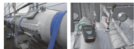
図3 吊橋主ケーブル送気乾燥システム Fig.3 Air injection system for main cables of suspension bridge
