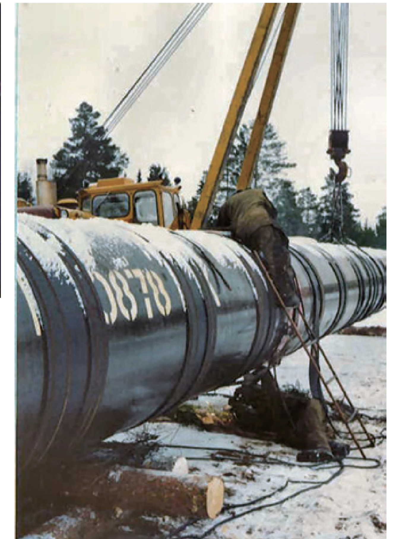
A Pipeline-Welding site in Russia where LB-52U is used for joining the girth joints in freezing weather
