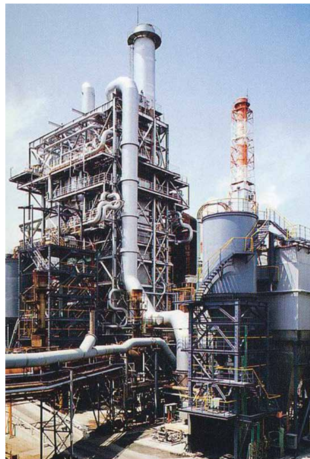
Coal-fired Steam Boiler Plant
