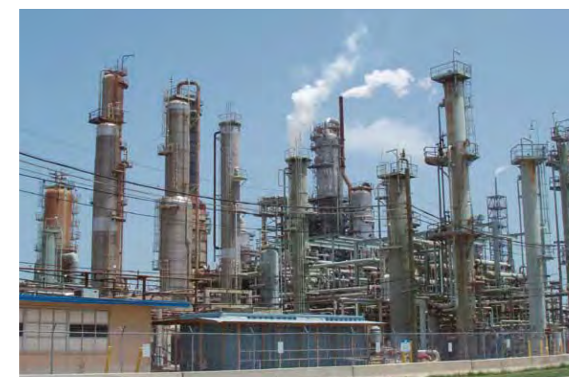
Chemical plant equipment
