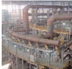
Rotary hearth furnace
