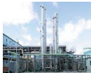
Biogas upgrading facility
