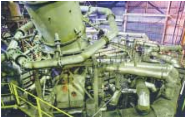
Photo 4 RHF in demonstration plant of ITmk3
