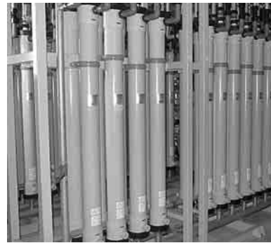
Photo 2 Membrane treatment system for water recovery
