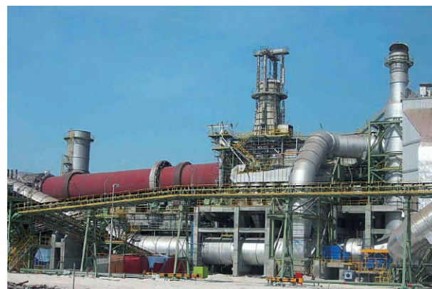
Fig.18 Photograph of GIIC No.2 pelletizing plant
