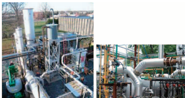
Fig. 6 Demonstration plant (left) and reactor (right)
