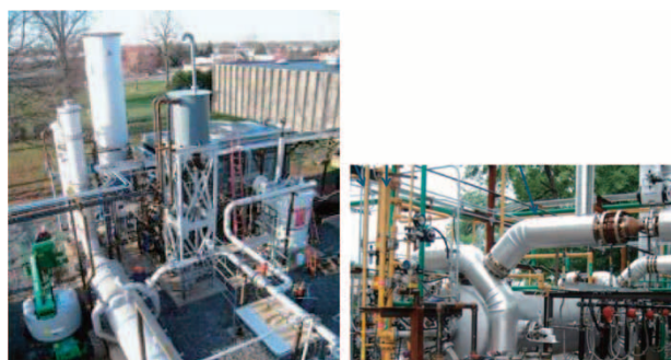
Fig. 6 Demonstration plant (left) and reactor (right)
