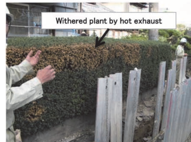
Fig. 1 Example of heat damage caused by mini excavator
