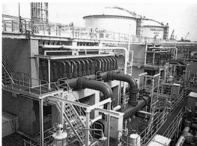
Fig. 3 — Cooling piping of the energy plants is one of the applications of NC-36L because of superior pitting corrosion resistibility against chloride ions.
