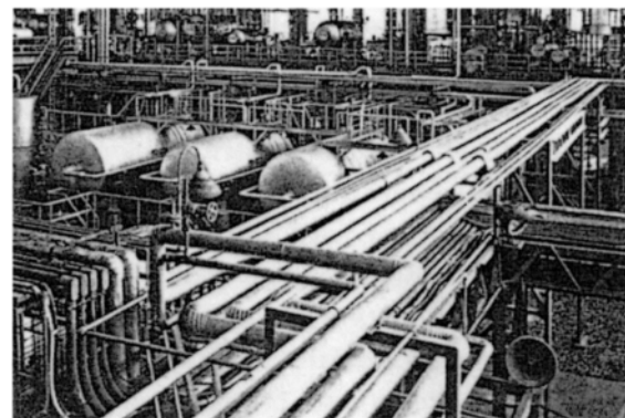
Fig. 1. TGS-2CML is more suitable for welding process-piping joints subject to short-time postweld heat treatment — thus lower temper parameter.
