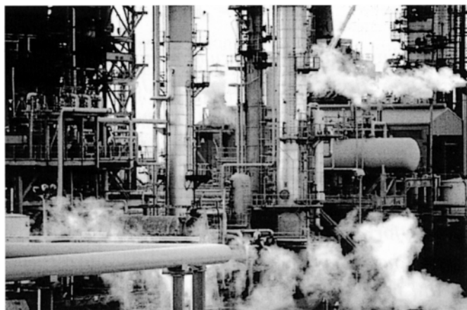
Photo 1. A refinery is composed of a variety of sophisticated equipment such as reactors, towers, heat exchangers, and pipelines.
