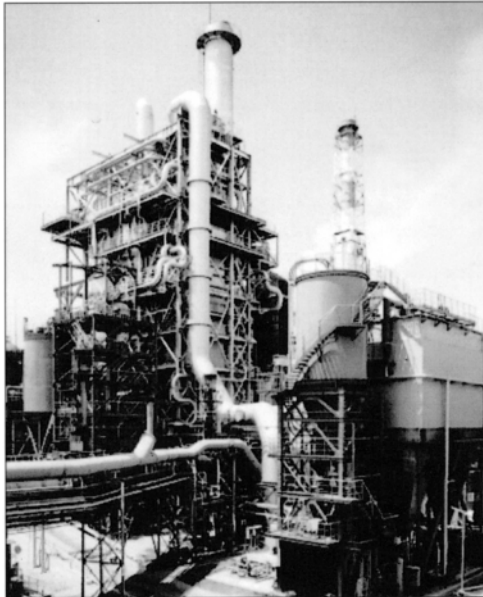
Photo 1. A coal-fired steam boiler consists of the sophisticated piping system fabricated with tens of thousands of tubes and pipes made from carbon steel, Cr-Mo steel, and stainless steel.
