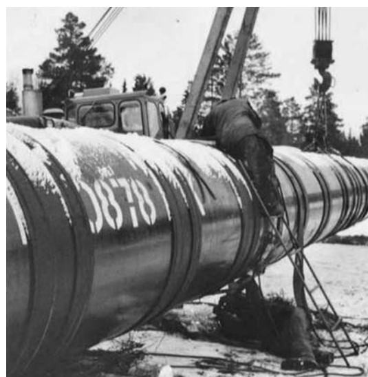
Figure 2: A pipeline-welding site in Russia where LB-52U is used for joining the girth joints in freezing weather.
