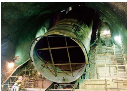
Figure 4: A unit pipe is joined to another unit pipe one by one in the inclined tunnel to construct the penstock (Courtesy of Mitsubishi Heavy Industries, Ltd., Japan).
