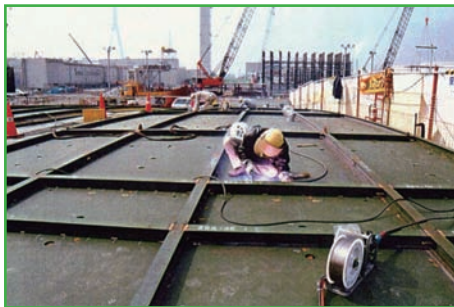
Figure 8: Horizontal fillet welding (2F) on the roof of an LNG tank is carried out with PREMIARC™ DW-N709SP flux cored wire.
