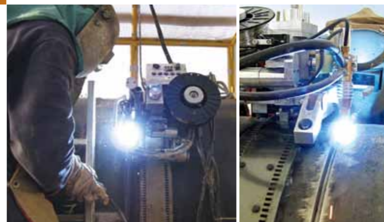
Figure 2: MAG welding by special girth welding machine. Photo courtesy of Pipeline Service S.r.l., Manufacturer of the Proteus FAP.
