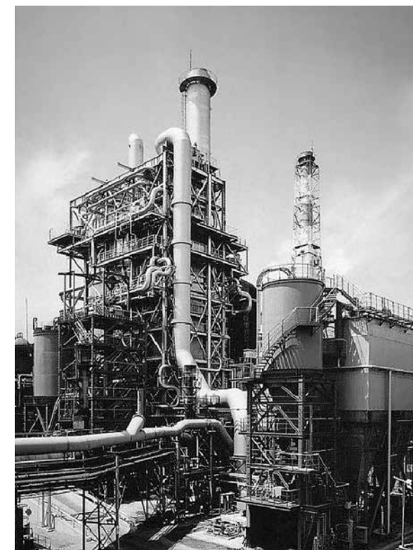
Figure 1: A coal-fired steam boiler consisting of the sophisticated piping system fabricated with tens of thousands of tubes and pipes made from carbon steel, Cr-Mo steel, and stainless steel.
