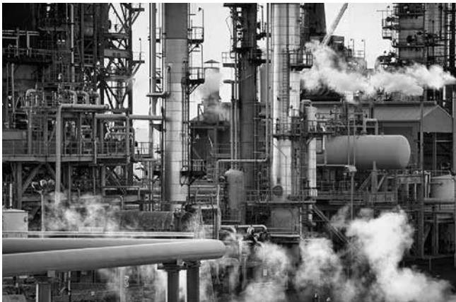
Figure 1: Refineries are composed of a variety of such sophisticated equipment as reactors, towers, heat exchangers, and pipelines.
