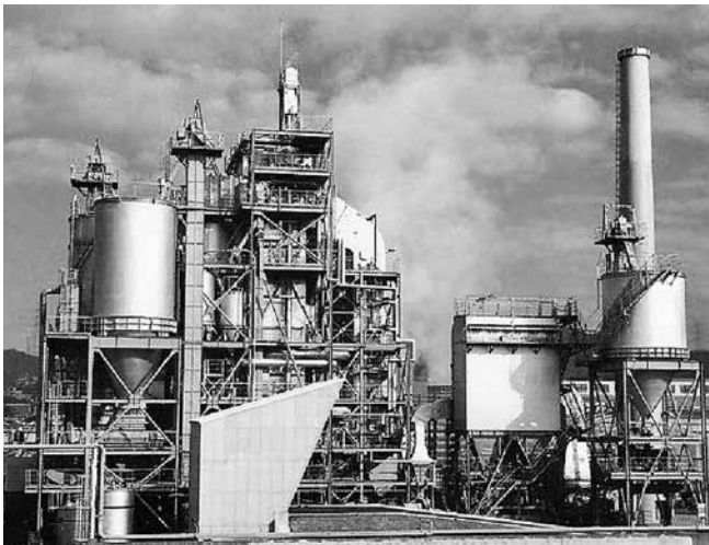
Heat-resistant low alloy steel is a main material for coal firing power plants.
