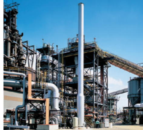
Pulverized Coal Injection Equipment
