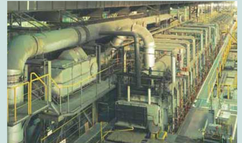
Roller hearth continuous annealing furnace
