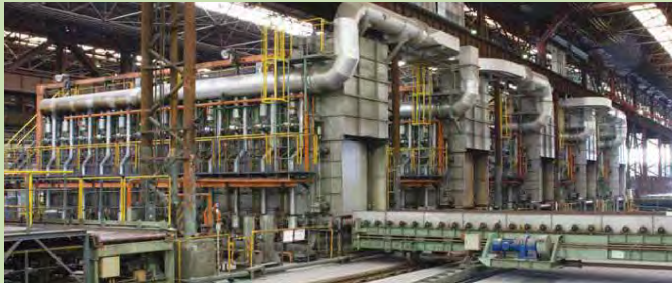
Heat treating furnace (Batch annealing furnace)
