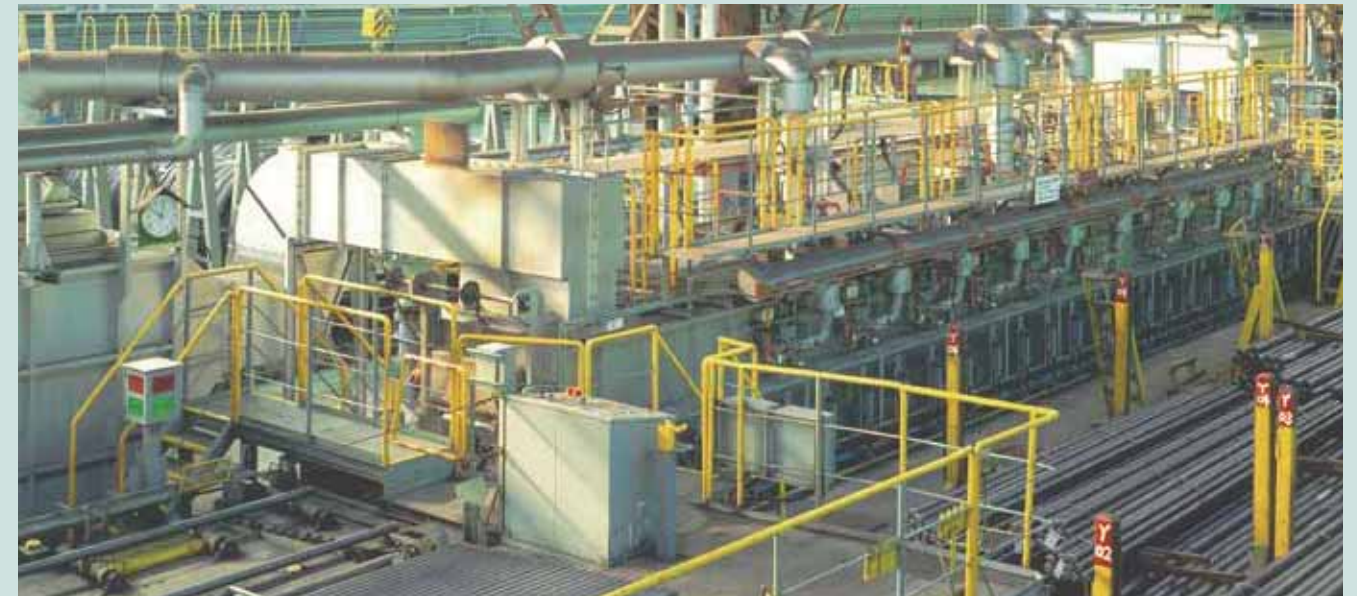
Roller hearth quenching furnace
