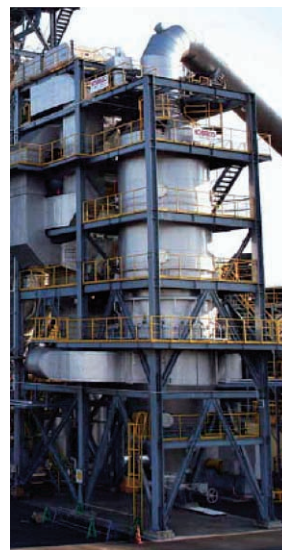
図12 新日鐵広畑製鐵所 FASTMET 3号機の排ガス冷却器 Fig.12 Exhaust gas cooler of 3rd FASTMET plant in Nippon Steel Hirohata Works
